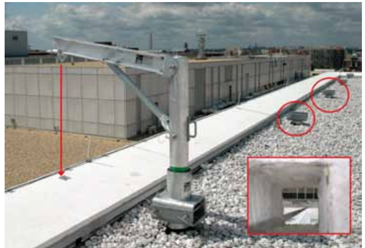
Davit pedestal bases were installed along the perimeter of this roof. The davit arm in the foreground can be moved to any davit pedestal base needed. Davits were installed to avoid loading the cornice. 5" x 5" sleeves were cast into the cornice to allow a suspended cable to pass through. This configuration maintains proper clearance between the suspended work platform and the façade.
