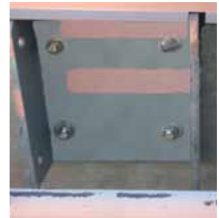
Wall davit pedestal base
